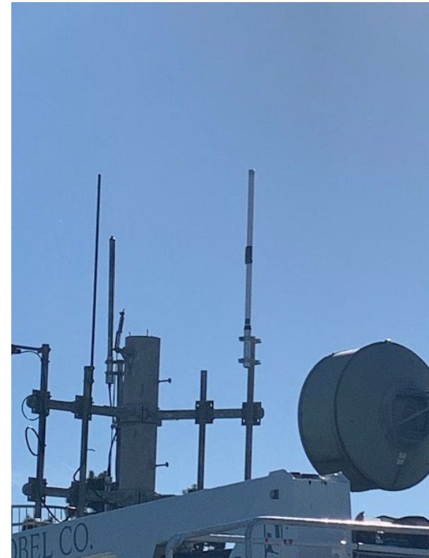
Pt Reyes TX and RX Antenna Installations
