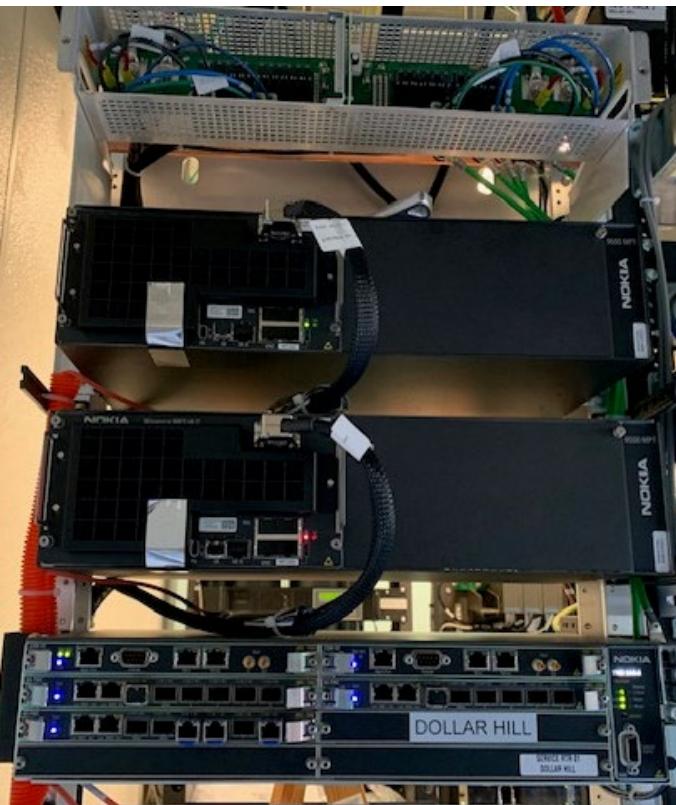
Dollar Hill MW Racks
