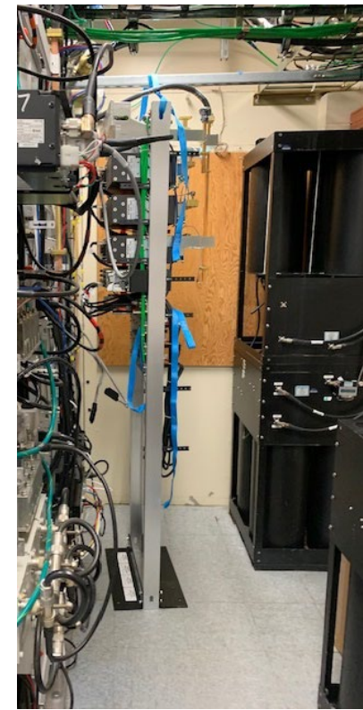
Big Rock MW Rack
