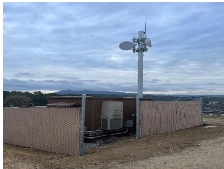
Skyview Terrace microwave site.
