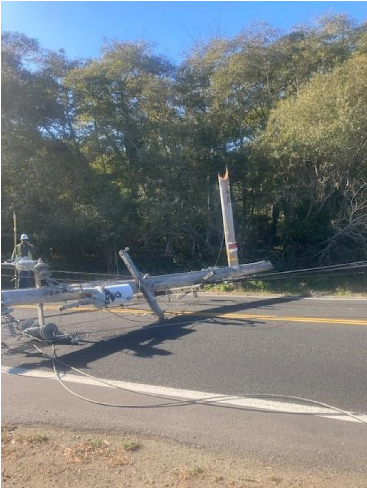
Cause of power outage when construction equipment was not secured to transport
