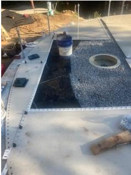
Tank #1 floor with drain
