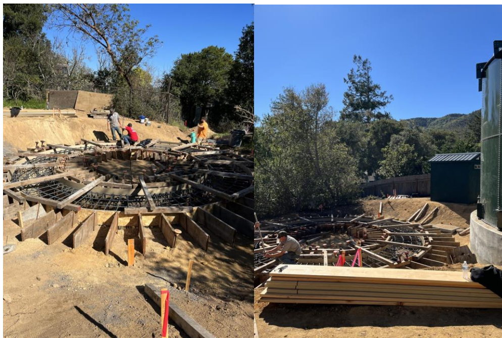
Tank # 2 footing framing for concrete pour facing east (L) and facing west (R)
