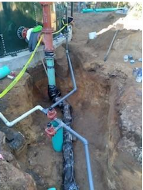
Tank #1 Outlet piping, east side of tank
