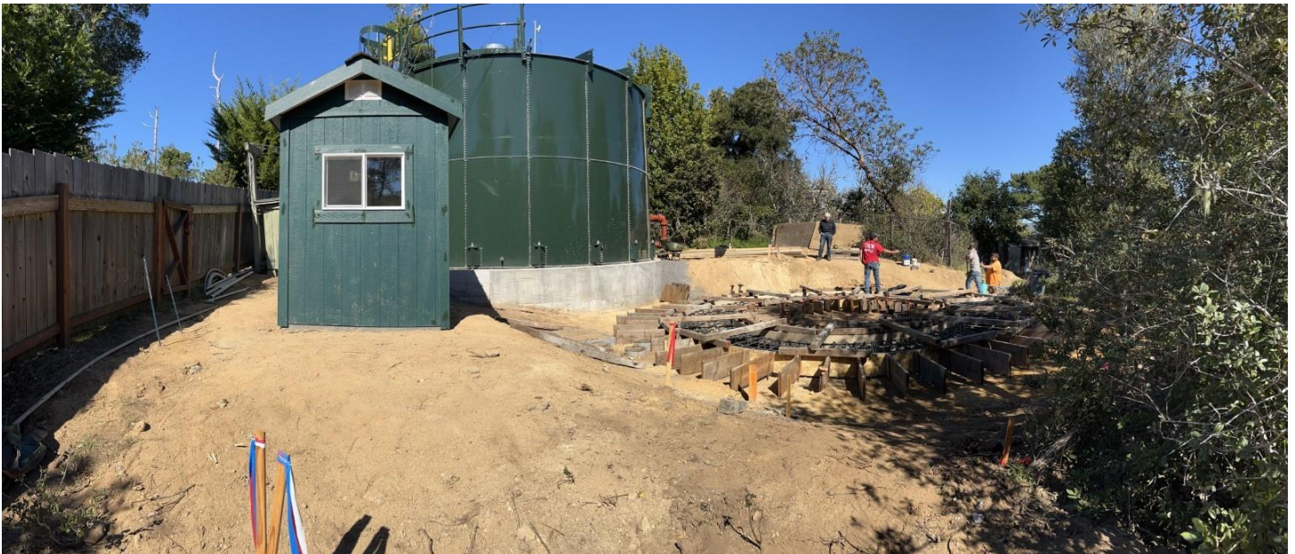
A Panoramic view of the Whole tank site looking north. There is the new shed for records and controls, the finished Tank #1 and the layout of the 2 nd tank foundation. Picture taken 2/17/2022.
