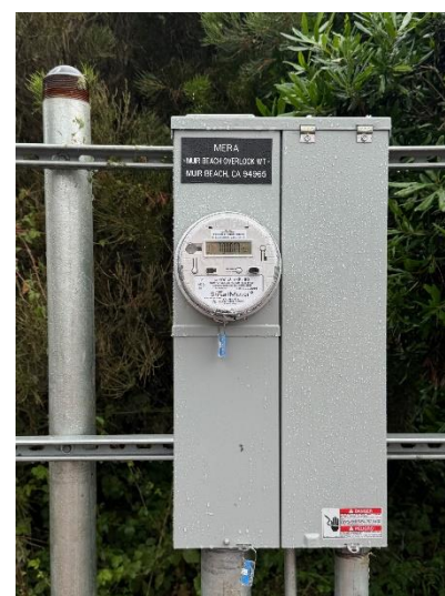
PG&E meter installed at Muir Beach Site.
