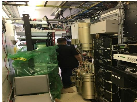
New radio equipment amongst the Gen I equipment at Point Reyes site.
