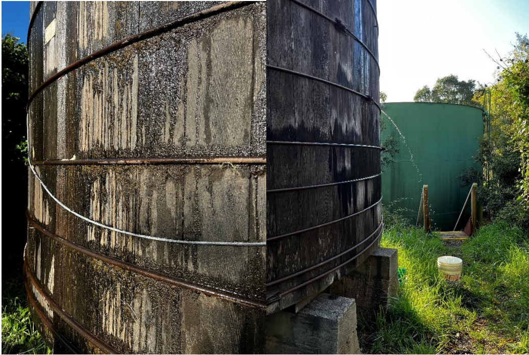
Above left: Colby redwood staves rot, bug damage. Right: active leak and stave rot.
