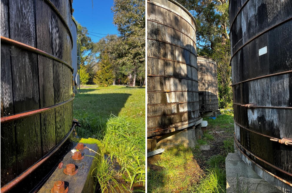
Above Left: Seahaven redwood tank active leak and rotted staves. Above Right: Colby redwood tank active leak and rotted staves.
