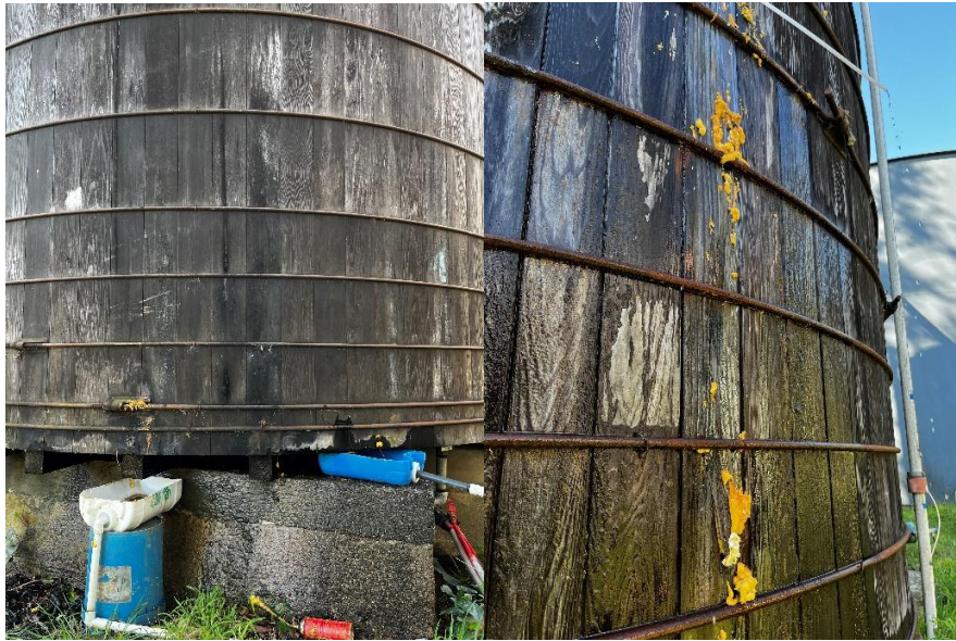
Above Left: Colby leaking redwood rotted staves, severe bug damage, active floorboard leaks.
